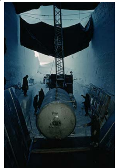
A crane positions Camp Century's nuclear waste tank. Photograph: W Robert Moore, National Geographic/Getty Images
